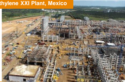
Ethylene XXI Plant, Mexico
