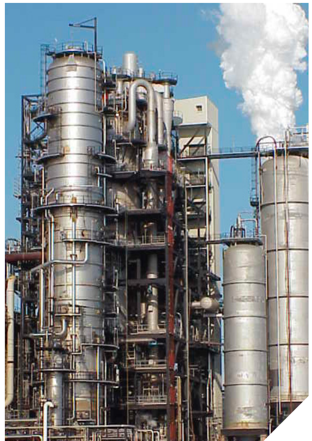
The TechnipFMC/Axens R2R cat cracker is designed for atmospheric residue feeds containing up to 8% Concarbon. This unit produces high yields of gasoline, diesel, and light olefins.
