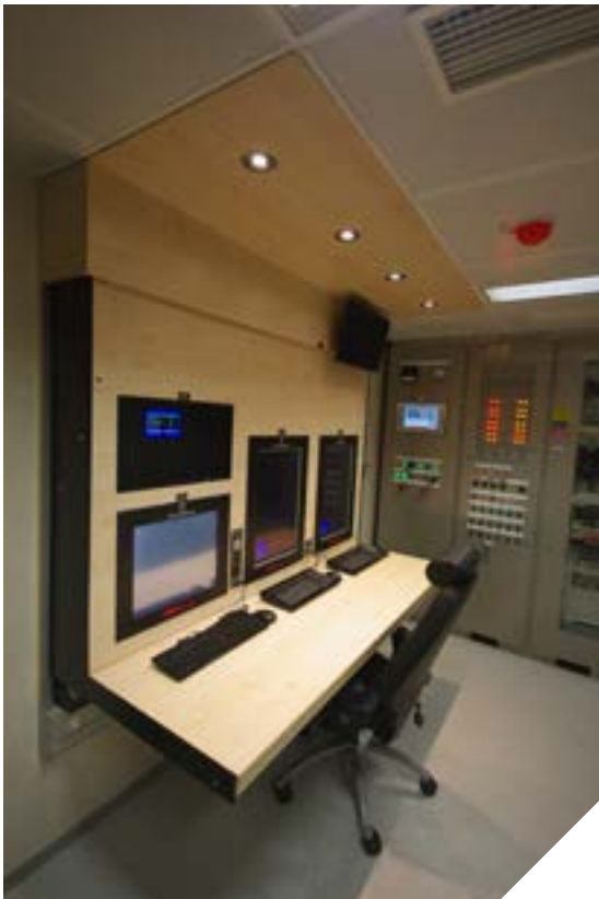
Master control station
